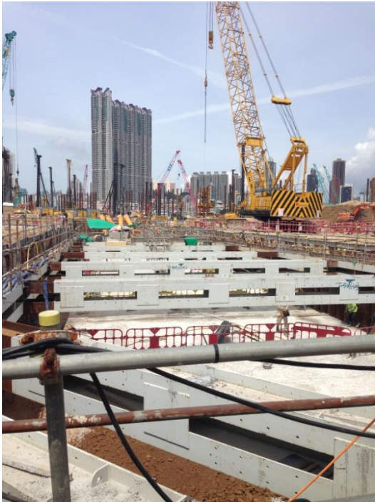
Fig.1 ELS works of the underground tunnel ventilation adit in Kai Tak site
