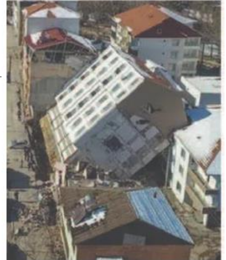
Effects of liquefaction, depicting a tilted building in the 2023 Turkey earthquake
