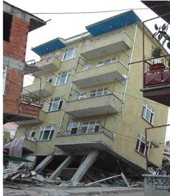
(Soft storey failure of infilled frame during the 1999 Izmit earthquake)
